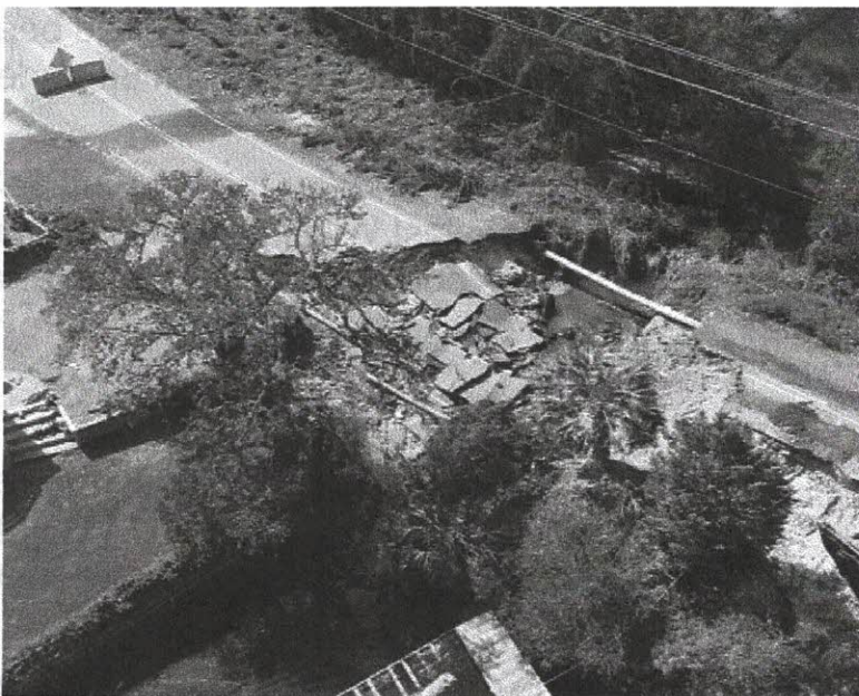
A view of the washout on Middle Sound Loop Road in Wilmington on Sept. 20, 2018 with pipes exposed. The challenges facing water system managers after storms come from both overflows and damage to infrastructure. Photo courtesy: NC Department of Transportation
